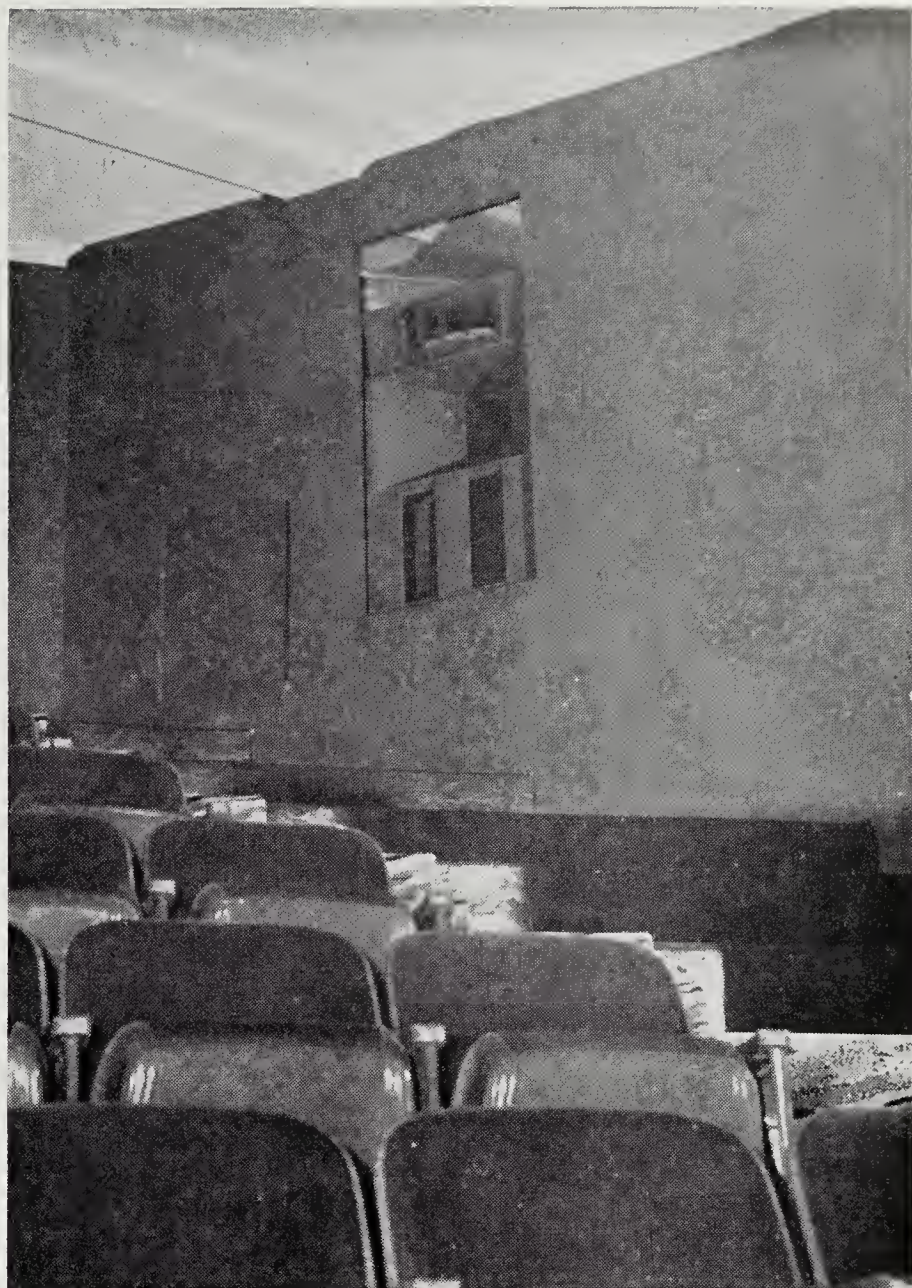
Shown is one of the four A7 Altec Lansing speakers, installed for "surround" purposes in the mezzanine of the Rivoli; they normally are used backstage.
